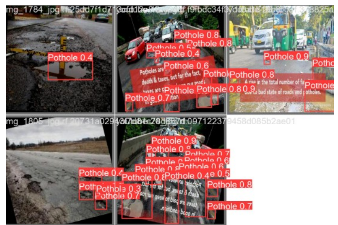
Fig. 5. Potholes captured and detected
