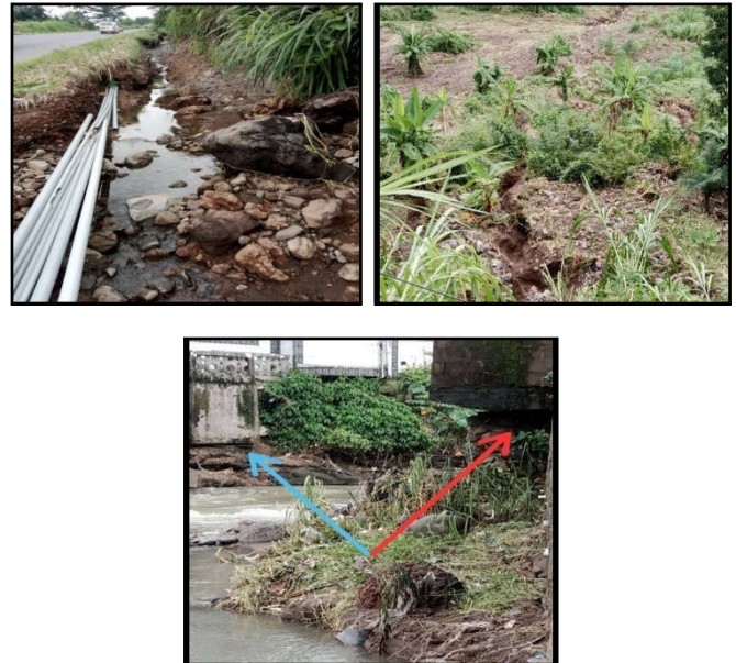
Figure 8. Artificial channels on main road and banana plantations, and eroded reclaimed land at Likomba Area Source: Fieldwork (2022)
